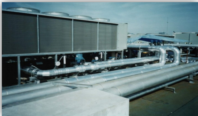
THE COGENERATION PLANT
